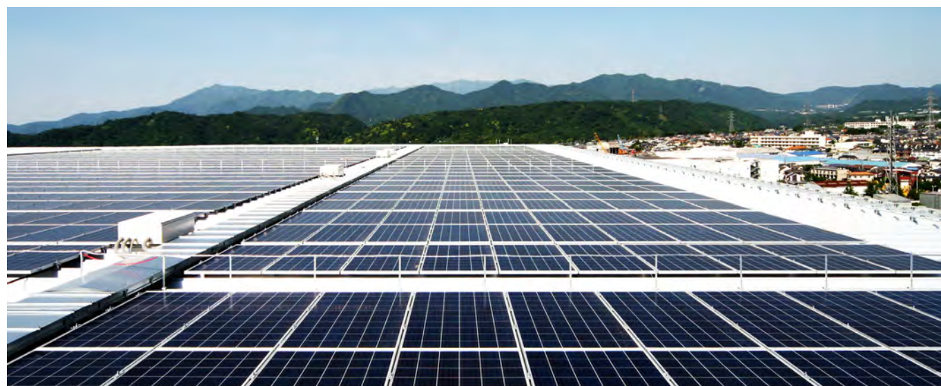
Solar power generation facilities
