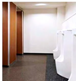
Water-saving by updating toilet equipment
