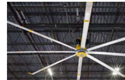
Large ceiling fan
