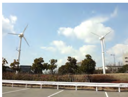
Wind power generation
