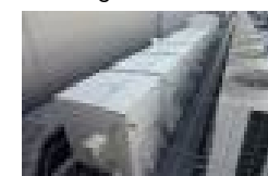
Ice storage air conditioning system
