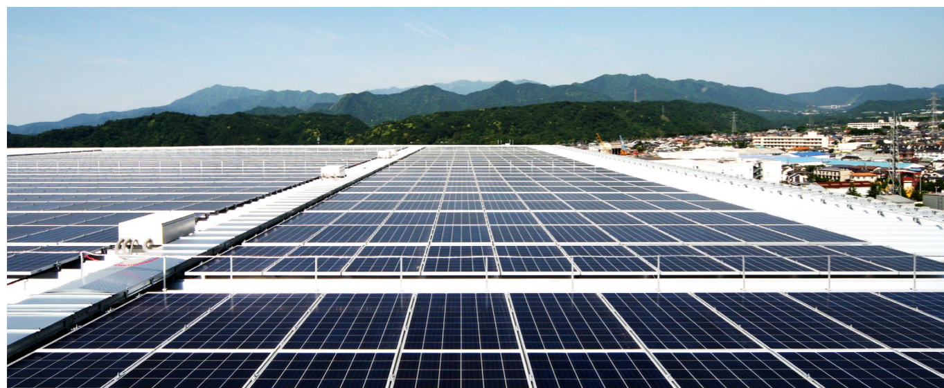
Solar power generation facilities
