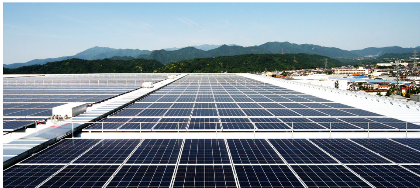
Solar power generation facilities
