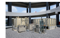
Groundwater Supply Equipment
