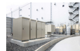
Emergency Power Supply
