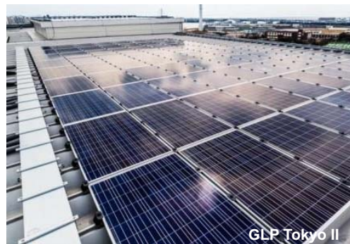
GLP Tokyo II Solar panel
