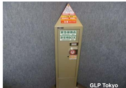
GLP Tokyo Emergency cabinet in elevator
